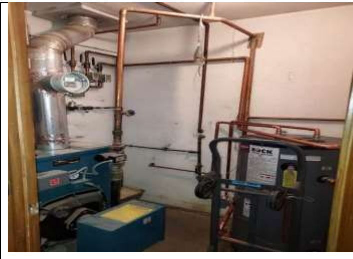
17. View of 497 Beaver Dam Road – Furnace
