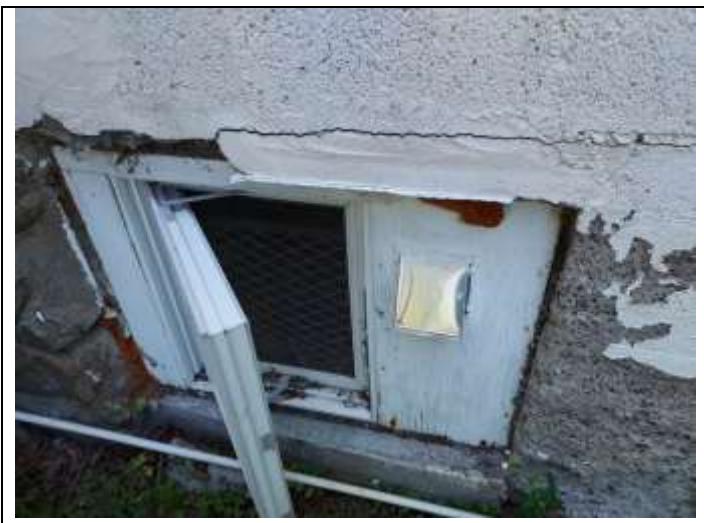
21. View of 497 Beaver Dam Road – Ext. Window Caulking
