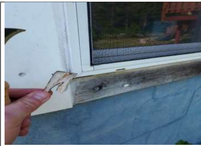
3. View of 355 Neelytown Road - Exterior Window Caulking
