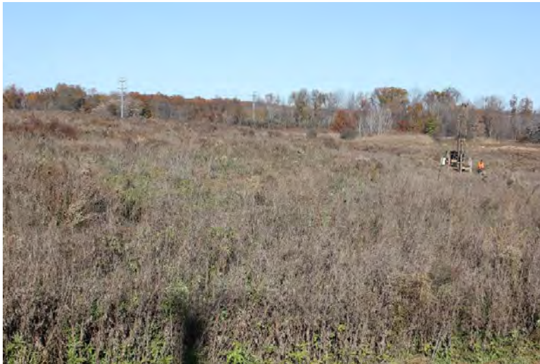
PHOTO 1. View facing northeast, from the shoulder of Dolsontown Road. The drill rig is working near the front right (southeast) corner of the proposed west warehouse. All photos were taken on November 10, 2021.
