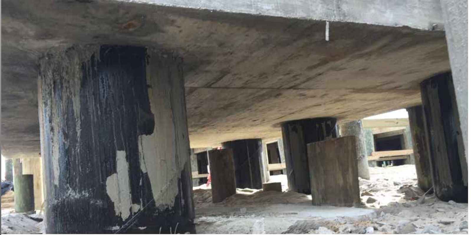
The lift tower's foundation required 24-inch-diameter steel pipe piles beneath the tower pile cap. Photo: Jim Elliott
