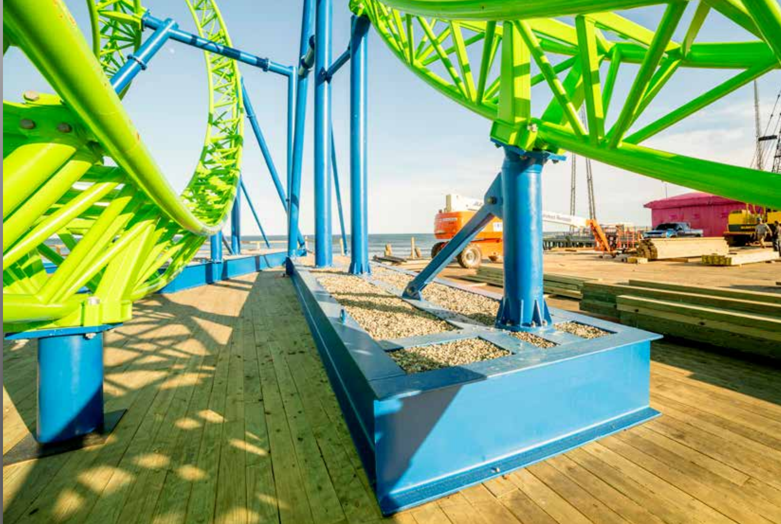
Steel-framed, car-sized pallets filled with heavy stone provide dead load counterweights to the coaster's large uplift and lateral foundation forces. Photo: Chris Spiegel Blurrevision.com
