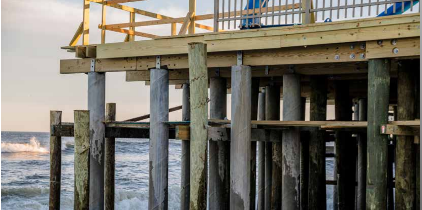
Steel sentinel pilings along the seaward side of the pier (prior to the removal of the timber piling sub-scaffolding) fend-off the extended hydrodynamic forces of moving water, wave action, and the large potential impact forces from storm debris “floatables.” Photo: Chris Spiegel Blurrevision.com
